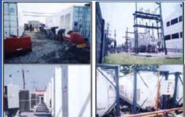
25MW Calapan Diesel Power Plant Occidental, Mindoro
